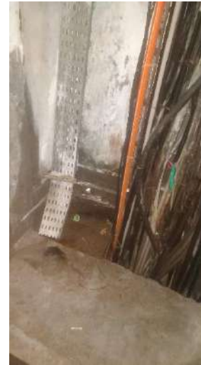
Image 7: Leakages in AHU rooms
