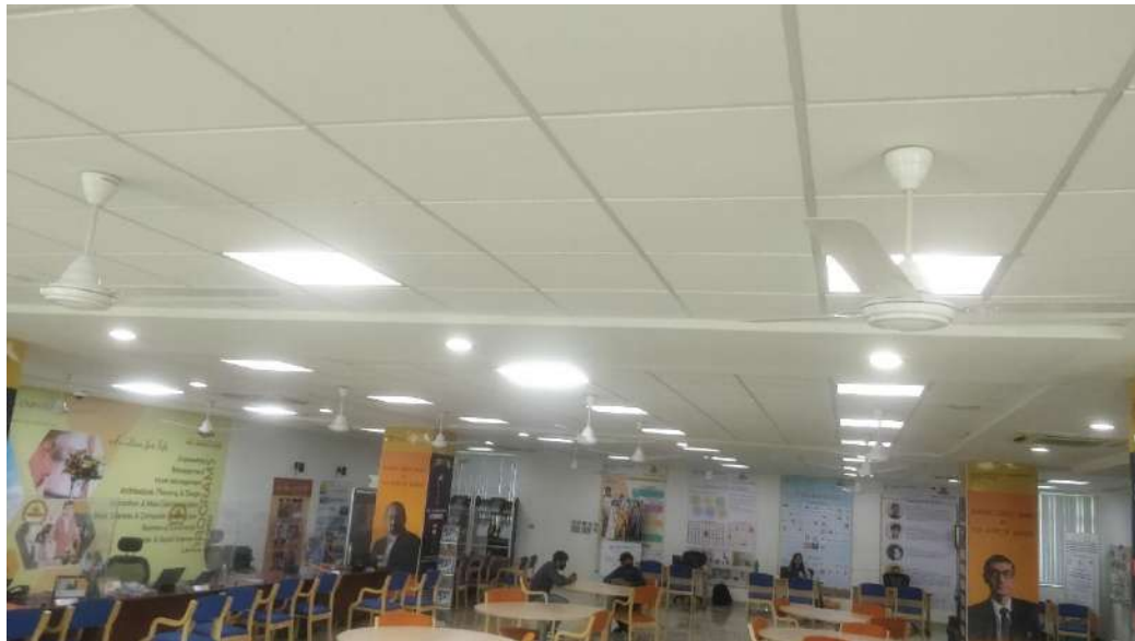
Image 1: LED Lighting Fixtures
